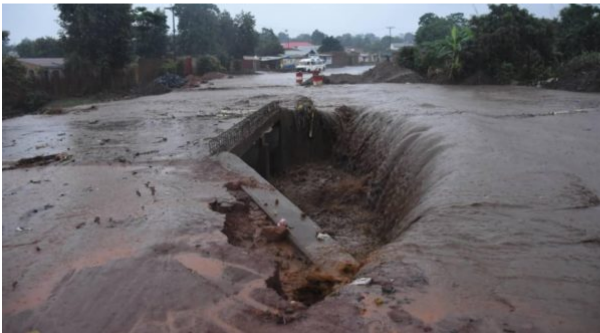
Kawale bridge damaged by the floods
