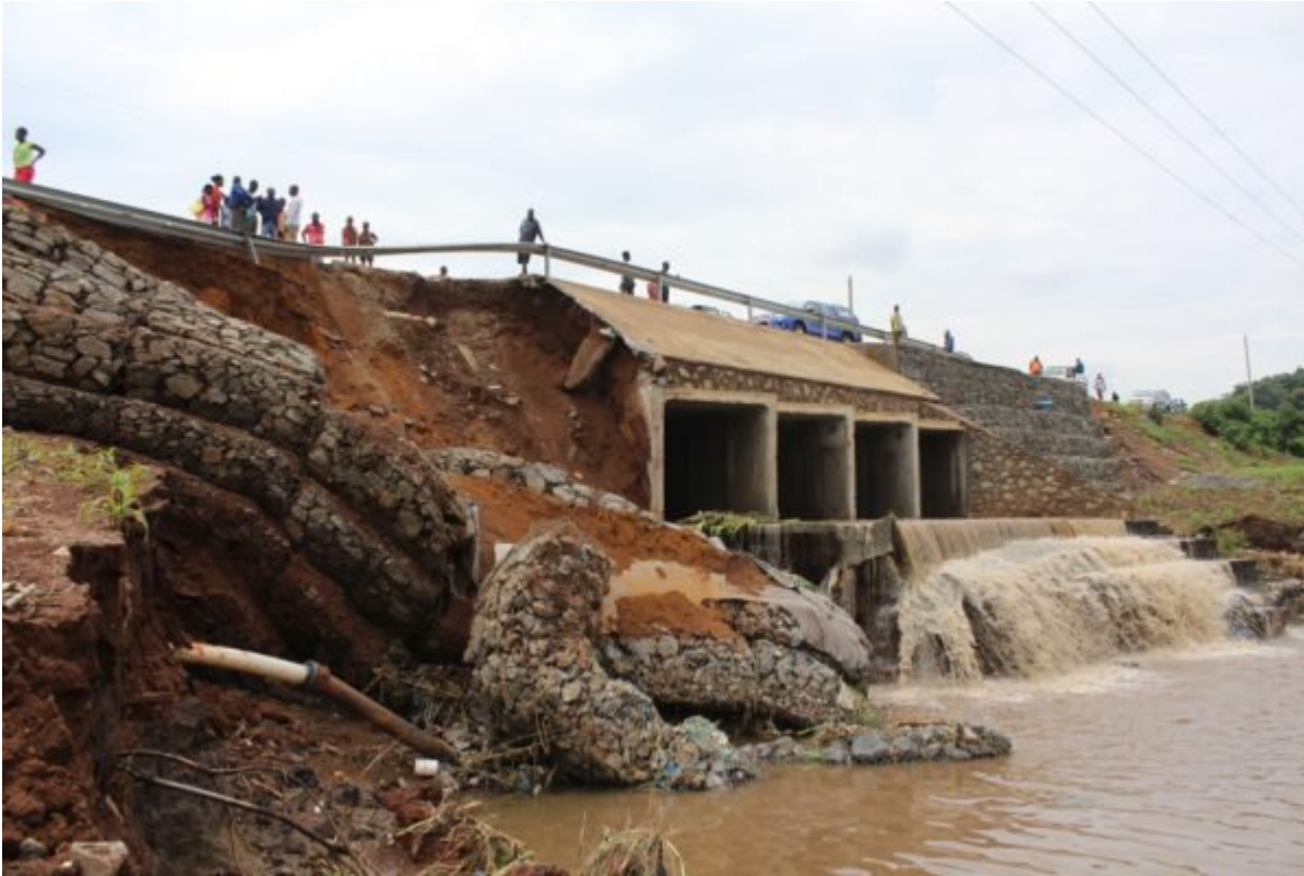
Chidzanja Bridge damaged by the floods
